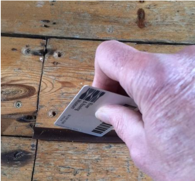
Gaps between floorboards
