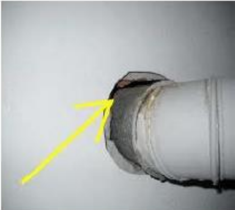
Pipework entry points
